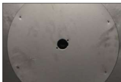
Internal cable fixing
